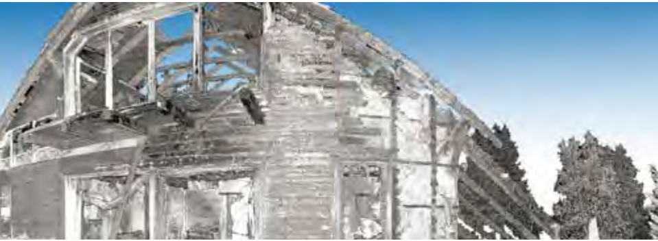
3D point cloud of a burnt restaurant
